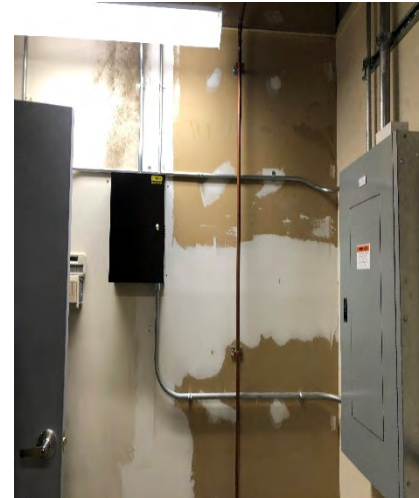
Figure 43: Stanley Security Solutions Panel - NE Data Closet
