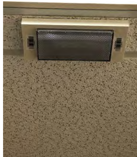
Figure 28: 32VDC Emergency Luminaire
