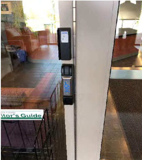
Figure 44: Card Swipe – Upper Level Vest. to Lobby Door
