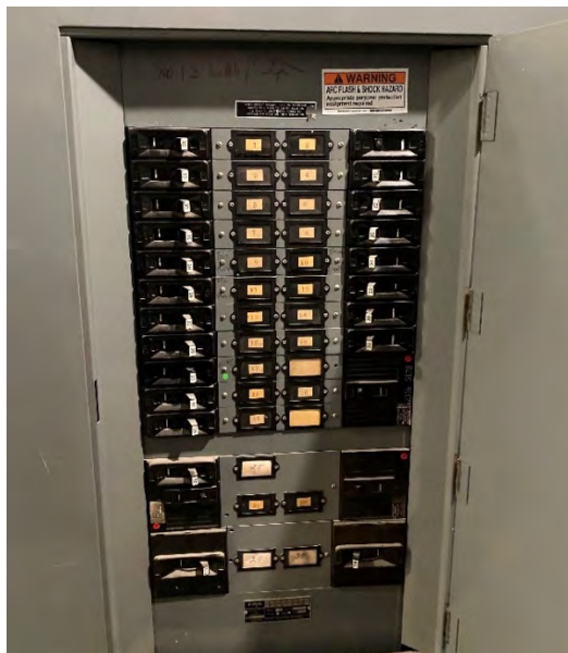
Figure 20: Lower Level Electrical Room – Typical Branch Circuit Panelboard
