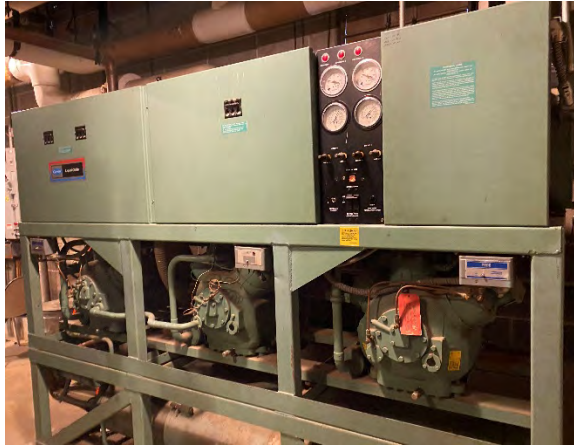
Figure 3: 77 Ton Water-Cooled Chiller in Mech Room
