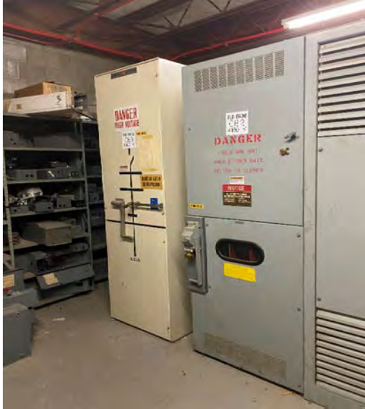
Figure 14: French Hall Unit Substation 5kV Selector Switch & Fuse Section
