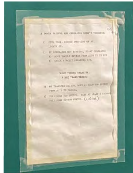
Figures 24: Automatic Transfer Switch with Operation Instructions for "IF POWER FAILURE AND GENERATOR DIDN'T TRANSFER"
