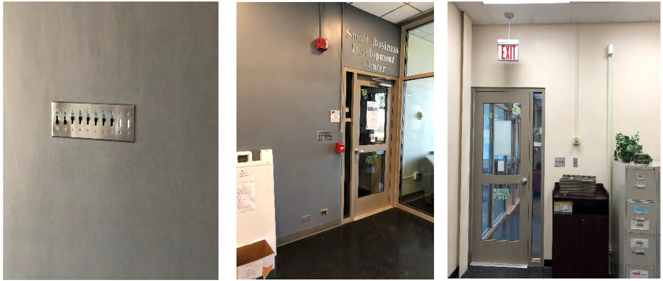
Figure 47: Examples of Lighting Switch Banks
