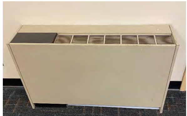
Figure 8: Typical Lower Level Console Fan - Coil Unit
