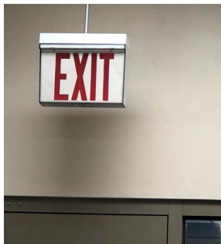
Figure 29: Exit Luminaire – Not Illuminated
