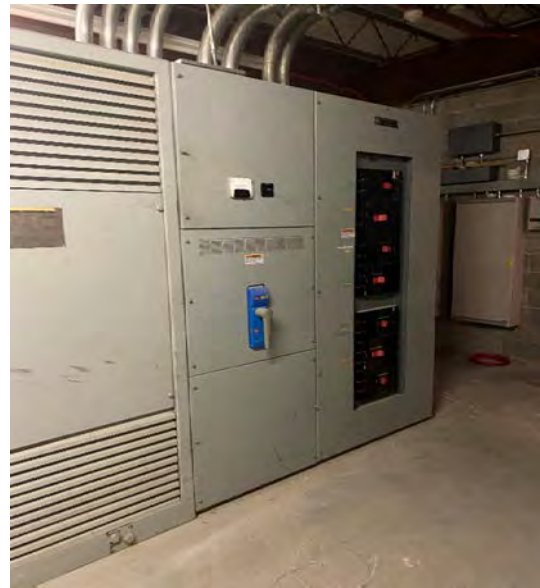
Figure 15: French Hall Unit Substation Transformer & Switchboard Section
