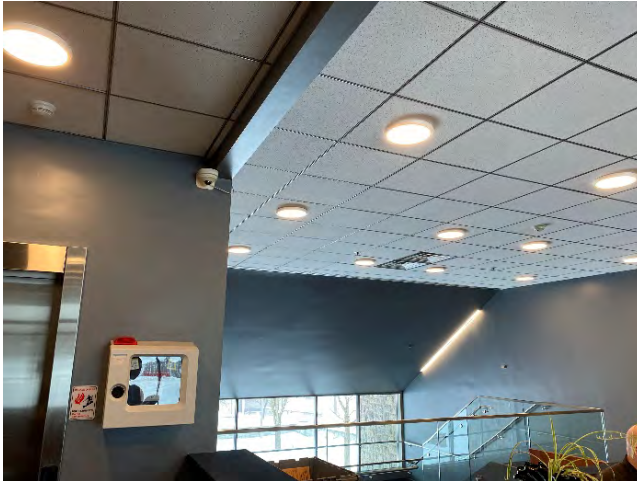
Figure 42: Security Camera – Upper Level Lobby Area
