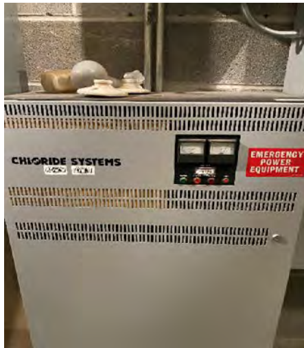
Figure 27: Emergency Lighting Inverter
