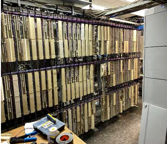
Figure 32: Analog Telecommunication System Serves the Entire SUNY Canton Campus
