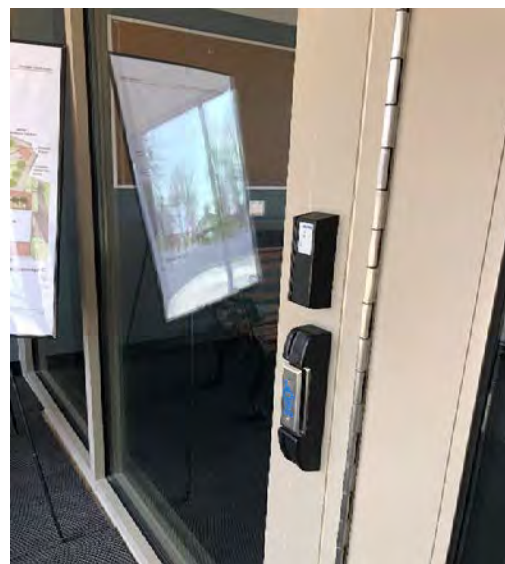
Figure 45: Card Swipe – Lower Level Vest. to Lobby
