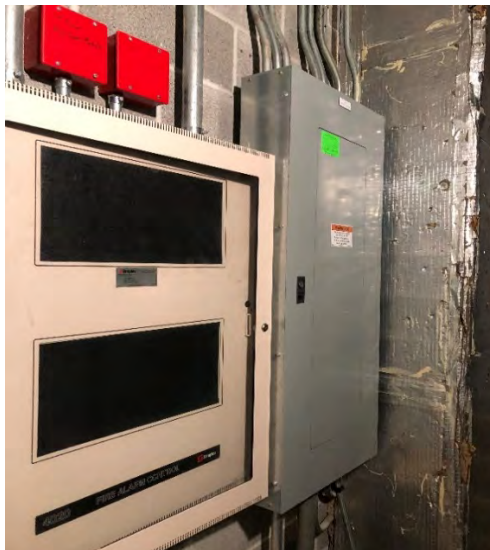
Figure 18: Upper Level Electrical Closet – Left Wall
