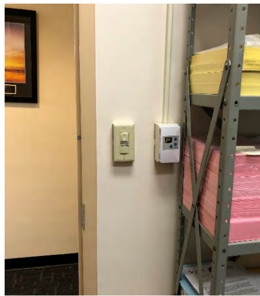
Figure 49: Vacancy Sensor - Upper Level Storage Room
