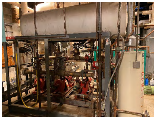
Figure 4: Existing Steam/HW Converter Station
