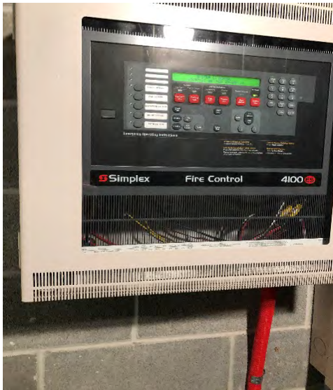
Figure 30: Addressable Fire Alarm Control Panel
