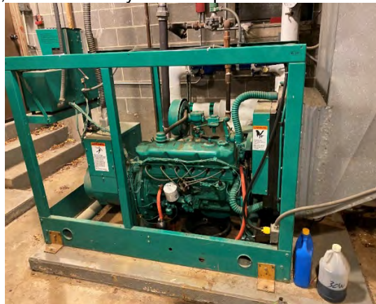
Figure 23: Telecommunications Room Back-Up Power - Natural Gas 25kVA Generator
