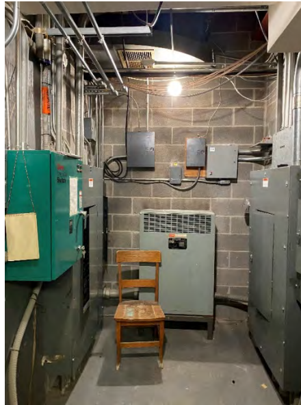
Figure 17: French Hall Lower Electrical Closet
