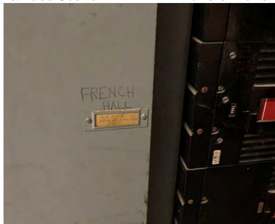
Figure 16: French Hall 700-amp, 480-volt, 3-pole Feeder Circuit Breaker
