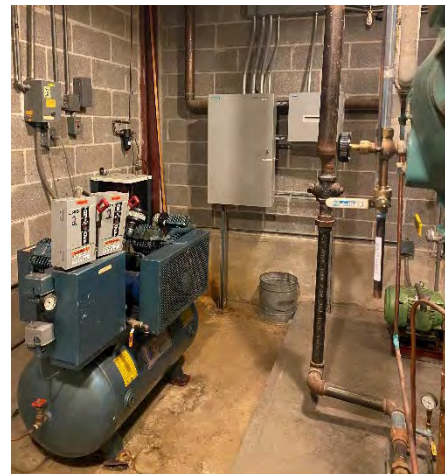
Figure 12: Control Air Compressor
