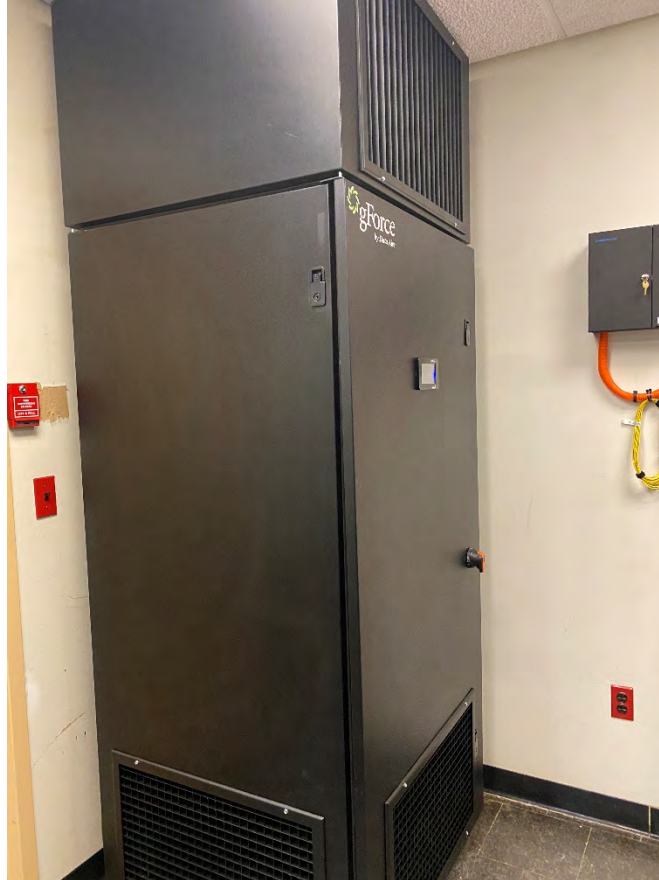
Figure 13: Computer Room Air Conditioning Unit
