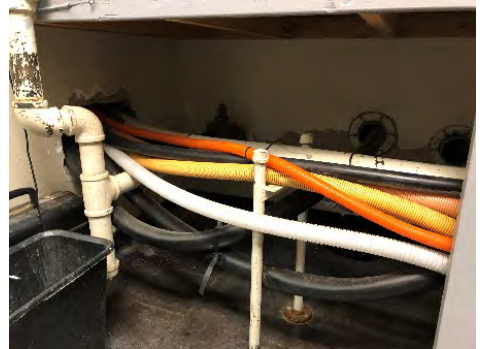
Figure 37: Telecommunications Cables to Vault
