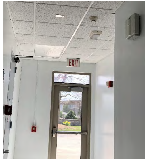
Figure 31: Fire Alarm Initiating Devices & Notification Appliances
