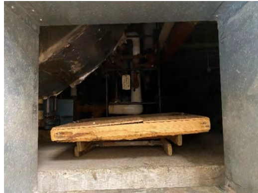
Figure 6: Access to 6,400 CFM Upper Level AHU
