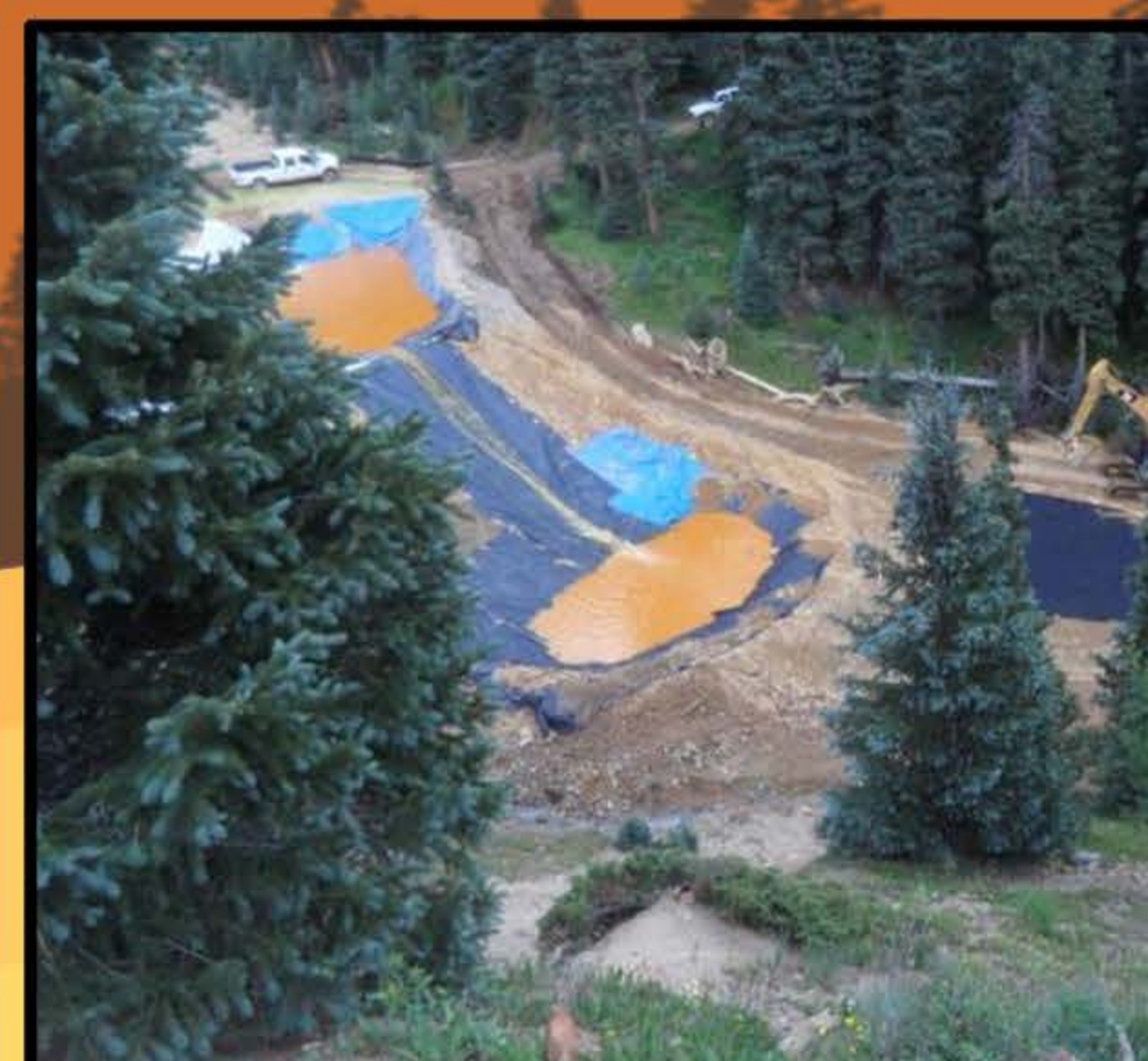
Figure 4. Settling Pools created by EPA for water treatment (flickr, 2015)
